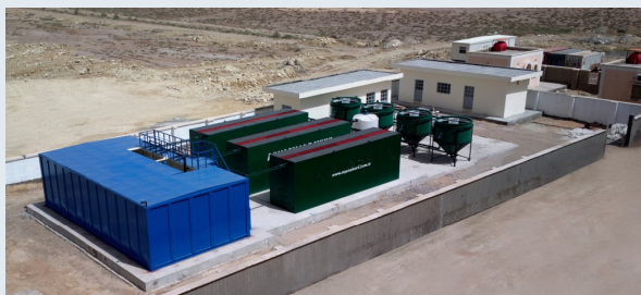
Containerized wastewater treatment plant operated with Mutag BioChip™, installed in Iraq in 2014
