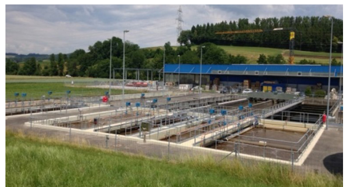
Fig. 3: Sewage treatment plant "oberes Surbtal". The biological treatment part of the plant consists of three identical treatment trains
