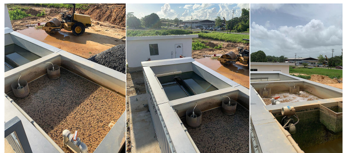
Fig 5: Containerized wastewater treatment plant operated with Mutag BioChip™, in Trinidad 2019
